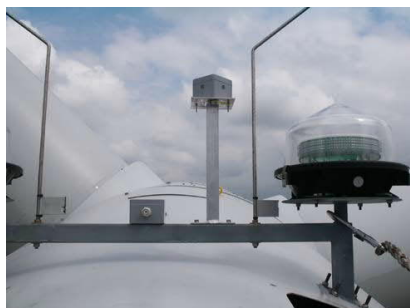
Figure 2. Sensor mounted to the top of a wind turbine nacelle.
